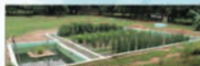
Constructed wetland for waste water treatment
